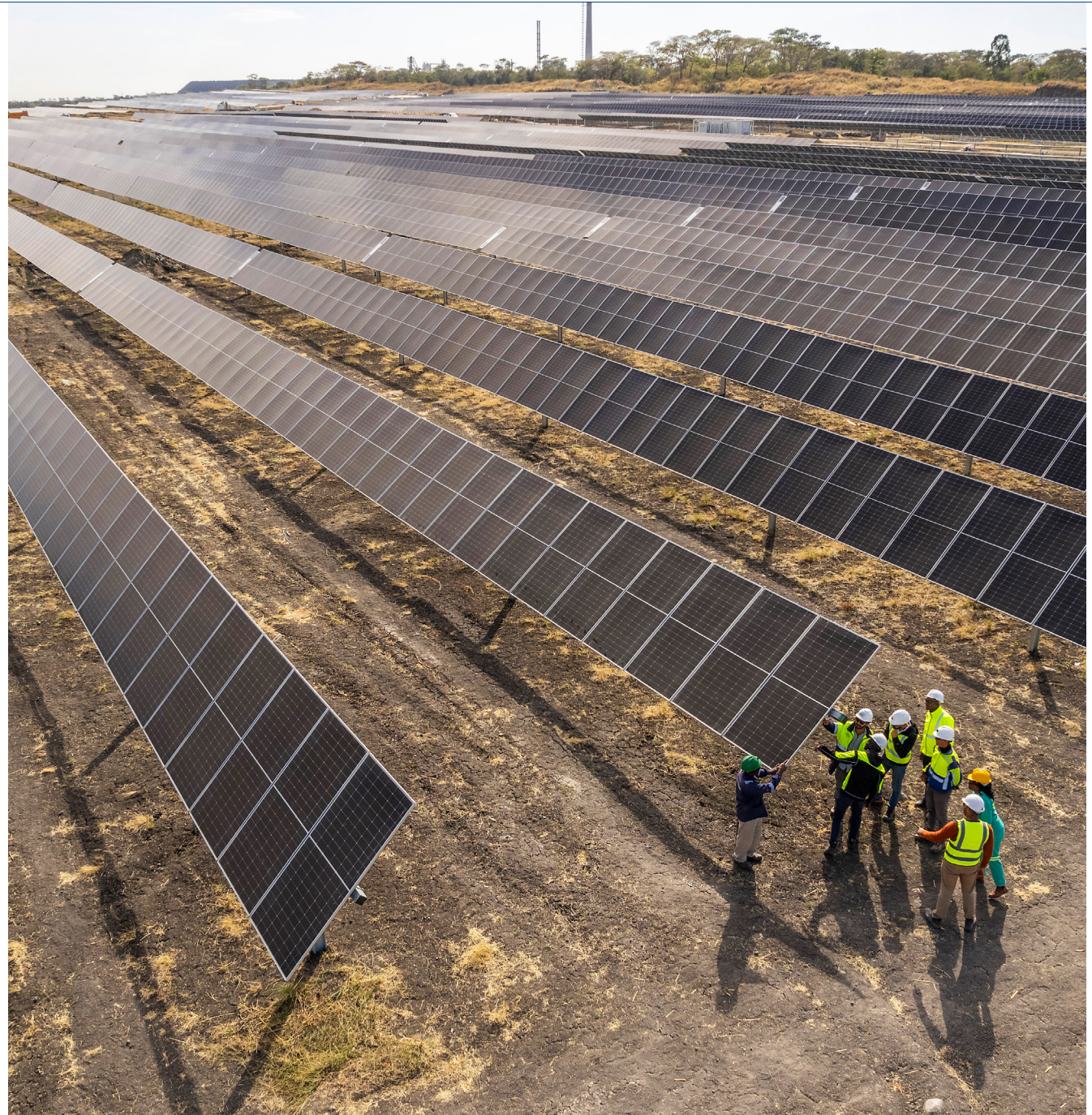
35MW solar photovoltaic (PV) installation at Zimplats
