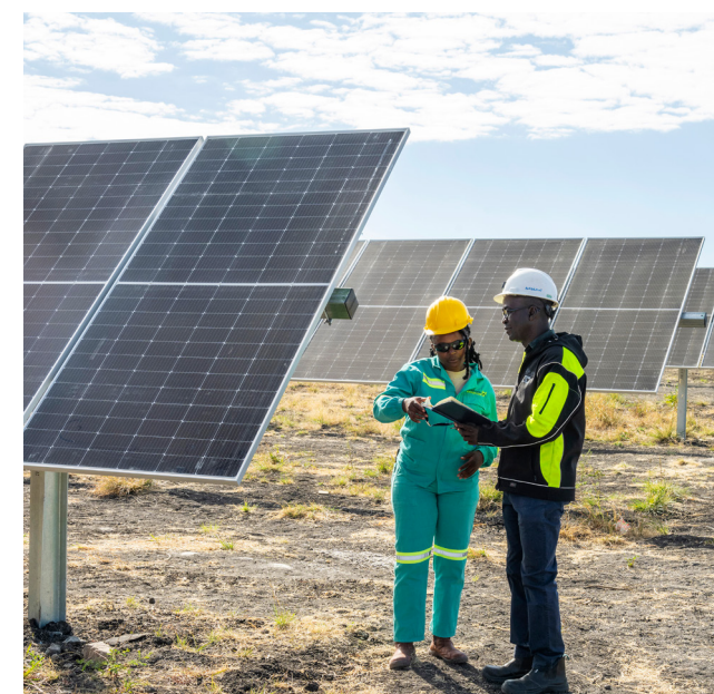
35MW Solar photovoltaic (PV) installation at Zimplats
