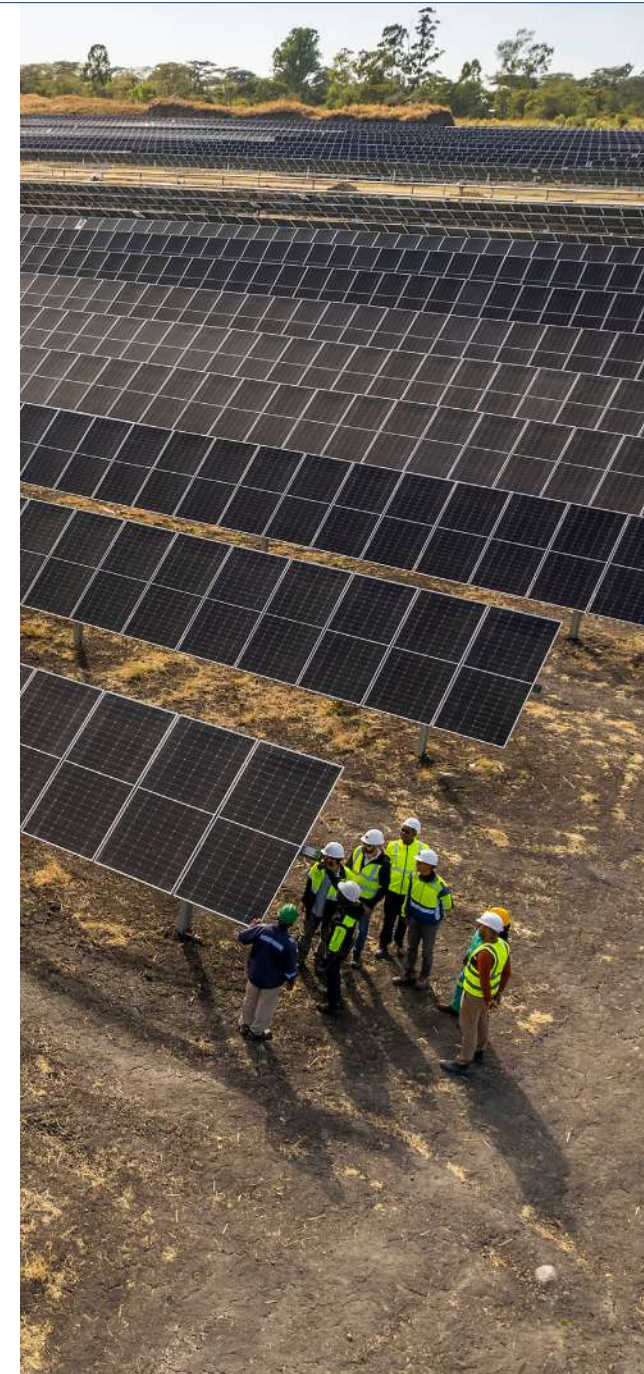
35MW solar photovoltaic (PV) installation at Zimplats
